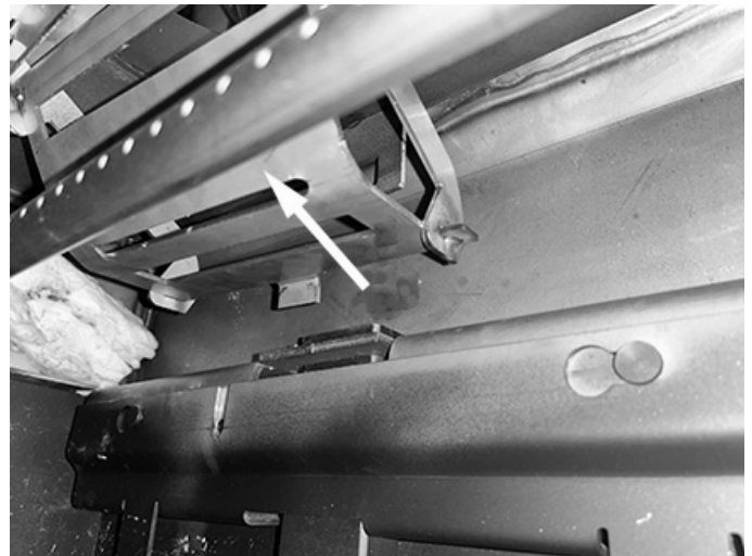
Figure 29. Remove Flue Gas Agitator
