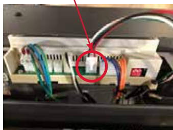
New Wiring Harness
