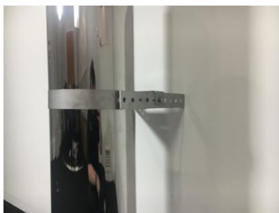
The brace wrap around the flue for firm and secure bracing
