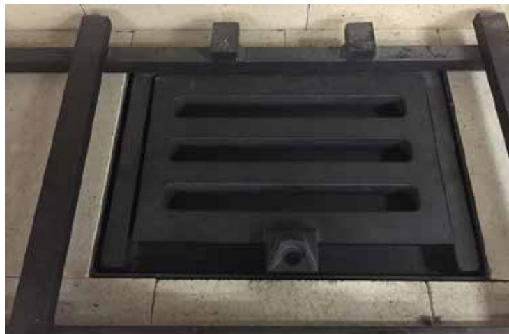
Figure 3) Ash Grate pictured in the fully-closed position.
